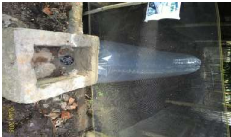
Gambar 3. Instalasi Biogas Digester Plastik
